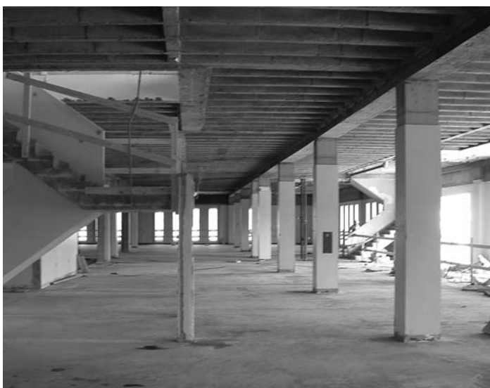
Top: Second floor construction of addition; middle: concrete forms will create the base for a strong second floor to hold compact shelving; above: existing building third floor during demolition.
